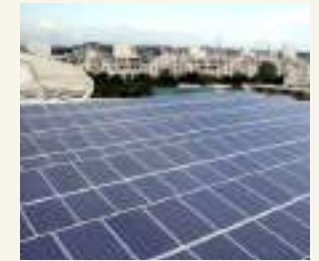
75 Kw Rooftop Solar system installed at MWC, Chennai
